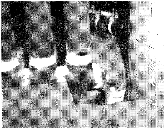
Figure 24. Cracking inside reformer furnace in elbow to vertical pipe weld caused by rotation of ring header below furnace wall.
